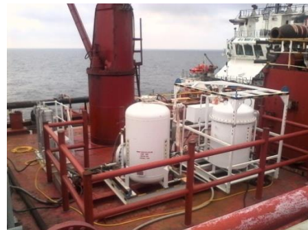
Picture of CHE equipment on the virini
